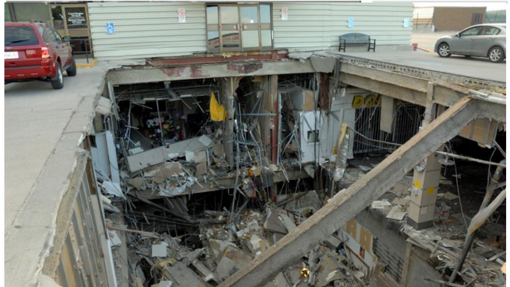
Infrastructure damage due in part to salt induced corrosion
